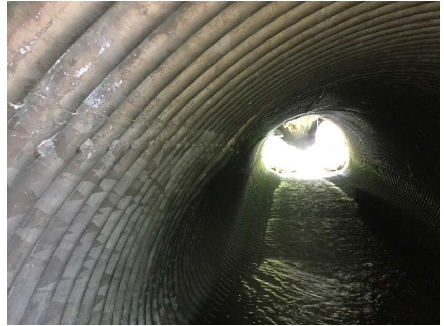
Minor damage noted near outlet
